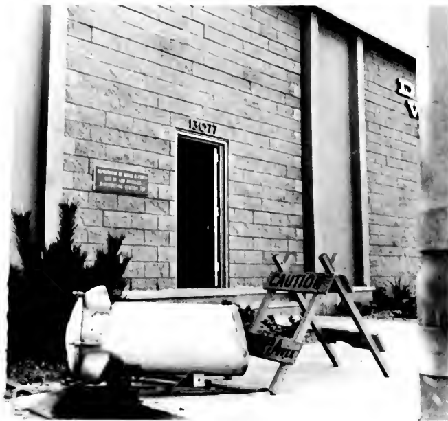
Photo 28. Damaged pole-mounted transformer on ground. Los Angeles Department of Water and Power photo.
